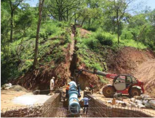
Water to drop ~80m and turbine to be positioned at this point.
