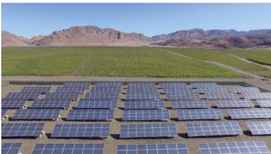
The 210 kW solar power unit at Silverlands Vineyards in Namibia.
